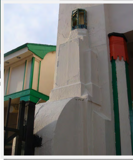
Building deterioration due to lack of maintenance
