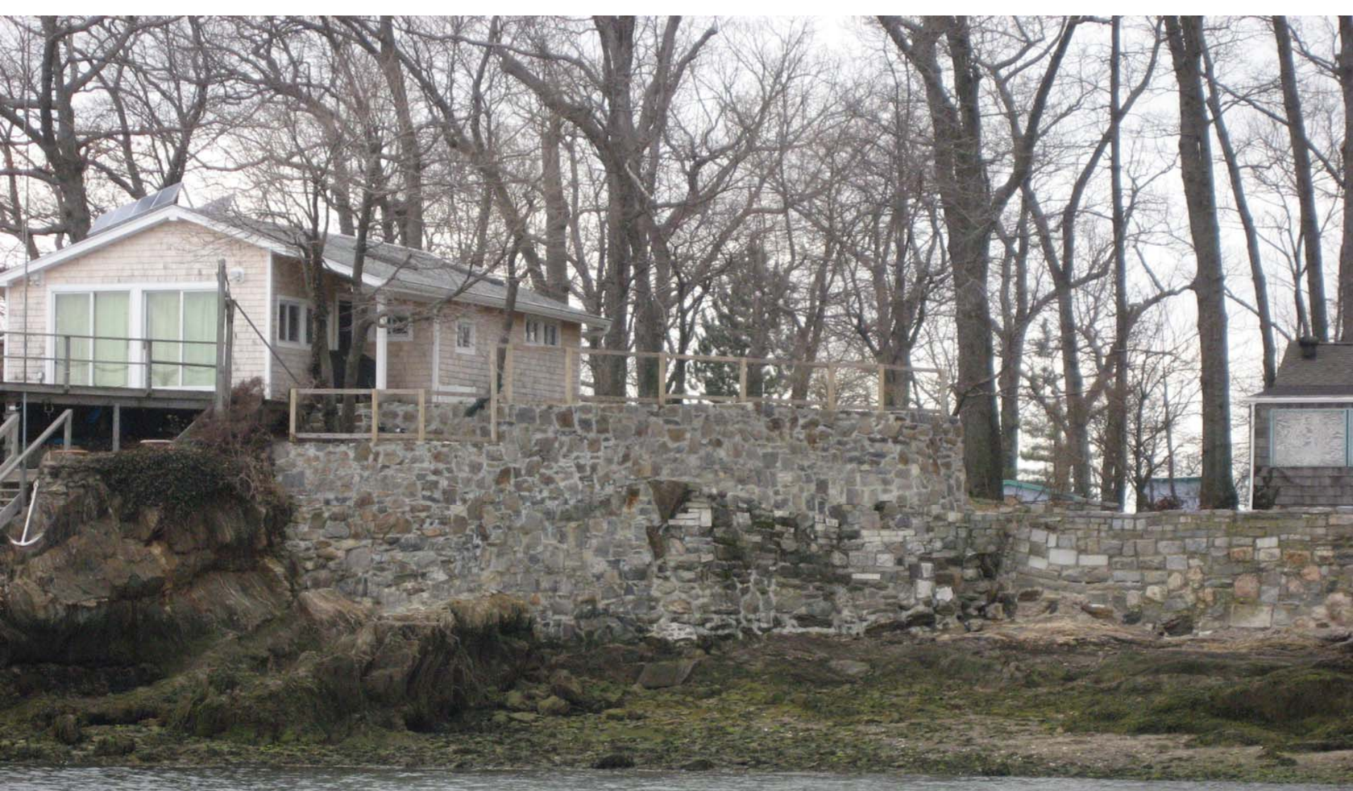
Illegally constructed sea wall
